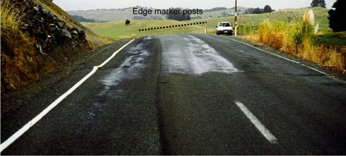
Figure 5 Edgeline, centreline and edge marker posts
